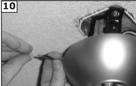
10 Make wire connections to power source using wire nuts provided. Make sure that no filaments are outside of the wirenut. After making the wire connections, the wires should be spread apart with the grounded conductor and the equipment-grounding conductor on one side of the outlet box and ungrounded conductor on the other side of the outlet box.
