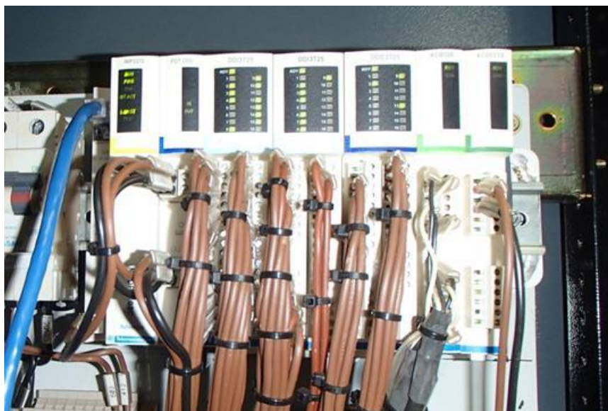
Figure 12 Advantys Remote I/O Module in VSD Sync Cabinet
