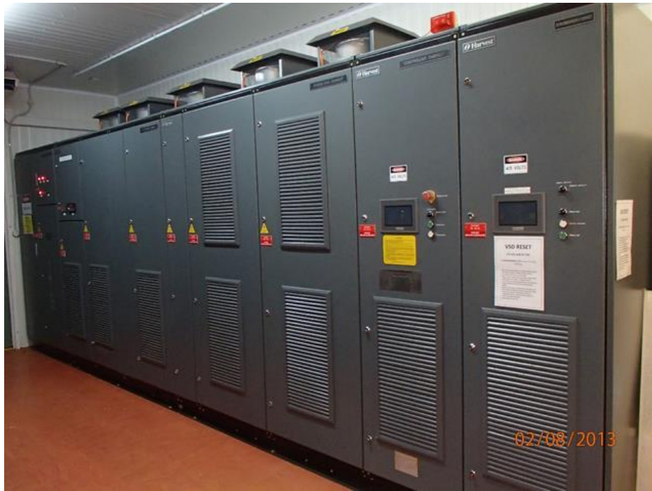
Figure 21 CV102 MO1 VSD and VSD Synchroniser Cabinet
