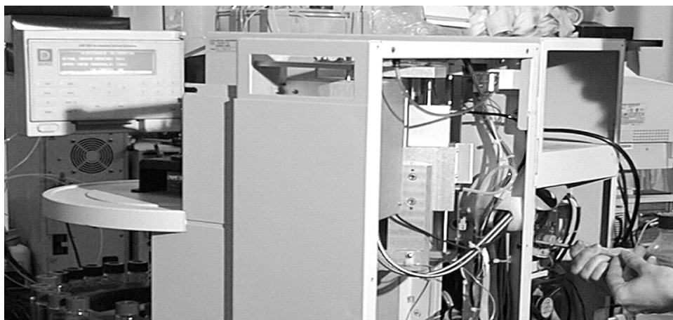
Figure 5-6. Accessing the Hydrocarbon Sensor
