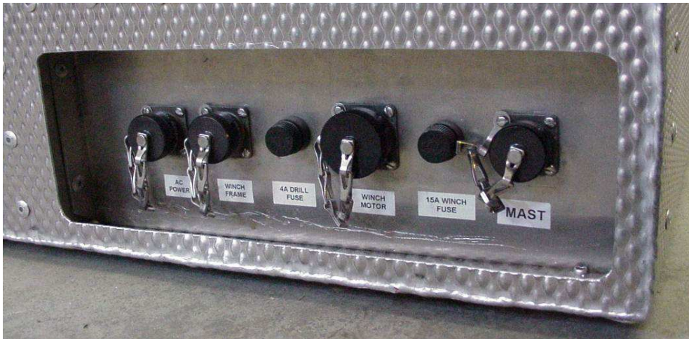
Figure 13 – Control Panel Back Panel
