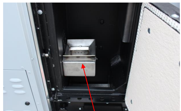
If the burner pot contains ash remove the pot for the holder and scrape the contents into a container. Also make sure that the air holes are clear. Carefully replace the pot ensuring that it is properly seated.
