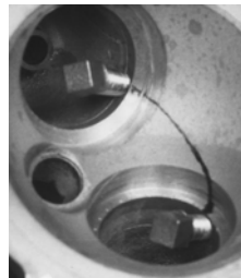
“Capture” the Crack
