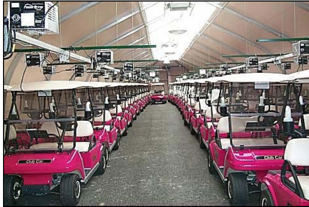
Figure 10 - Golf Cart Charging Units
