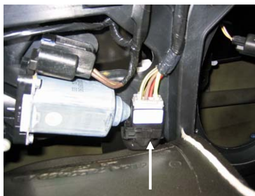
Recommended location to relocate switch
