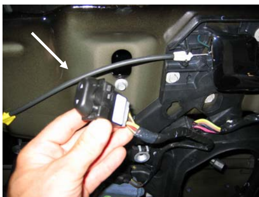
Remove window switch and reconnect. Wire tie switch in safe location.
