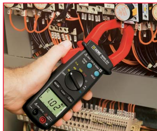
Clamp-On Meter Model 514 measuring primary current on a machine control system
