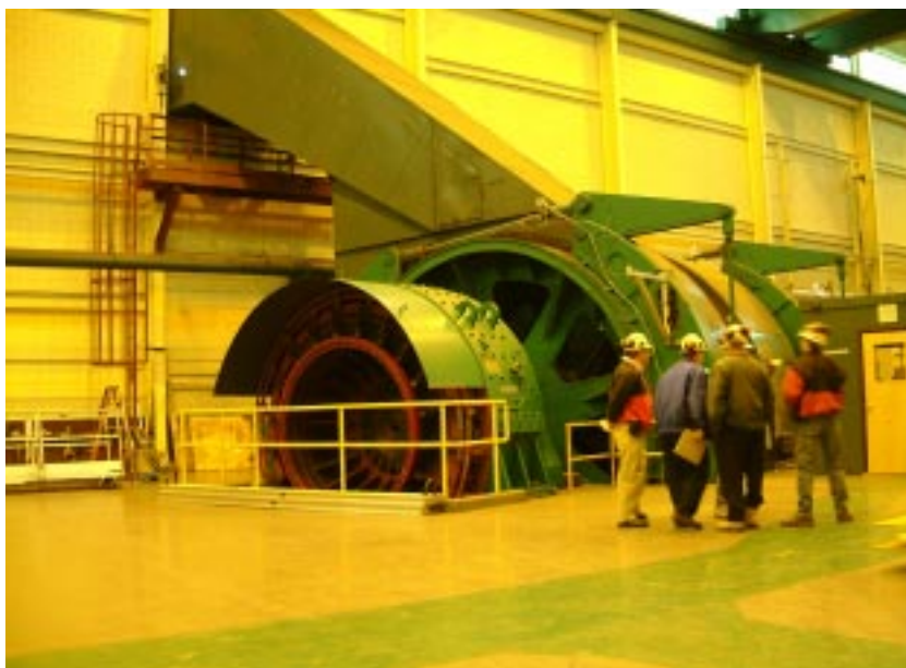
The Inco Creighton double drum hoist with existing DC motor.
