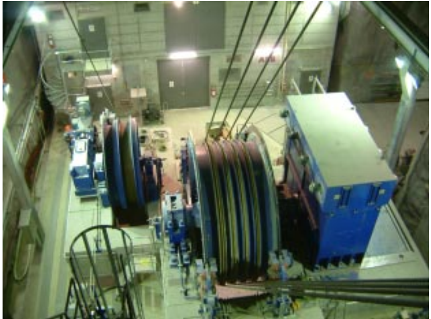
The hoist chamber at the Sedrun installation.
