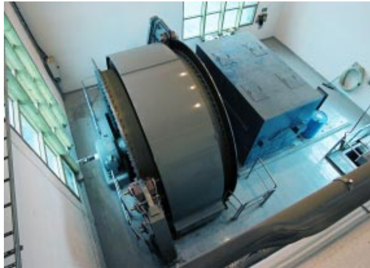
The hoist room at the Pyhasalmi Mine.
