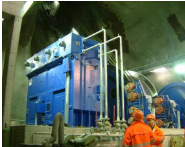
Water cooled 4 200 kW synchronous motor at the St. Gotthard tunnel.
