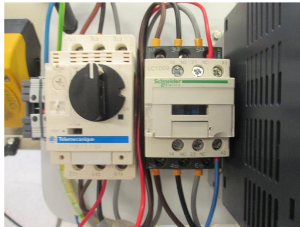
Figure 4.6 - Circuit breaker and thermal overload relay
