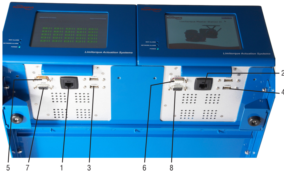
Figure 4.3 - Master Station Front Panel Connections
