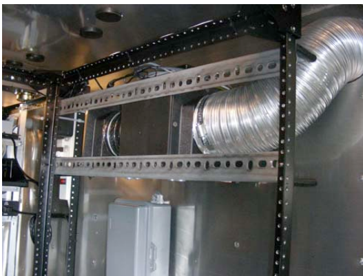
The forced air fan box enclosure mounted to the side of a rack in the MVSAT-120's front equipment compartment
