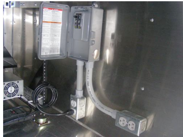
AC Distribution / Breaker Box
