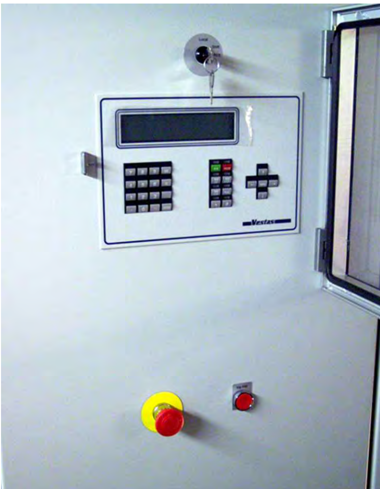
Picture 4 Emergency stop button at nacelle controller (pos. 4, Figure 1)
