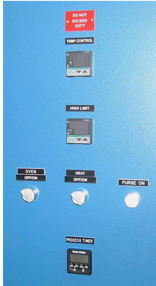
GAS HEATED CONTROL PANEL
