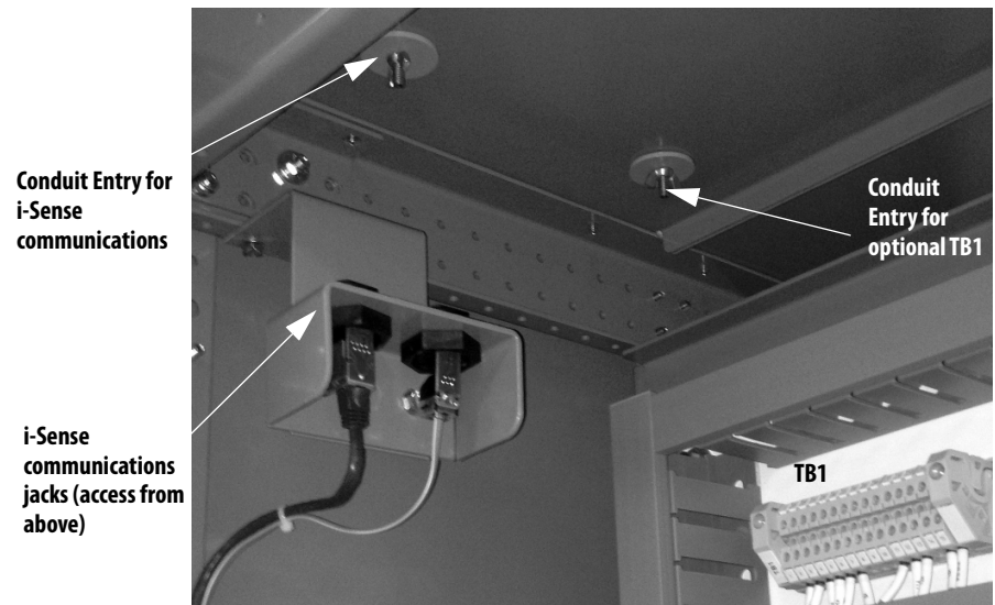
Figure 9 - Communications Conduit Entrance view from within upper switchboard compartment
