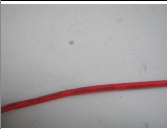
119 mark on internal wire
