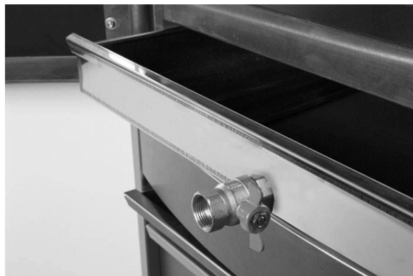
Drain valve closed. (Handle vertically)
