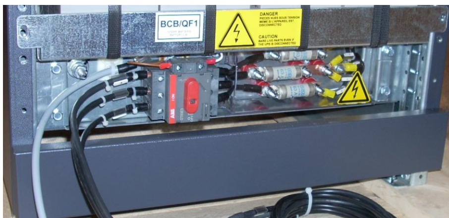
Picture 21 – Battery circuit breaker and fuses
