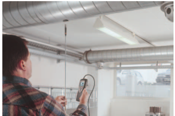
testo 416 helping to adjust supply air
