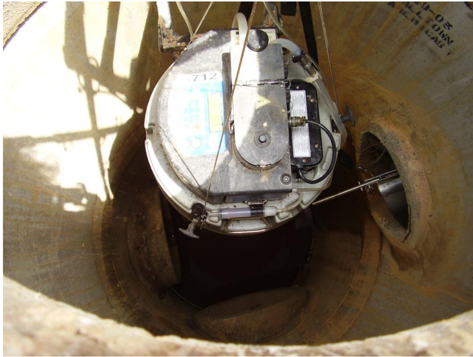
Figure B-1. Automated sampler placed in manhole using hanger and spring ring
