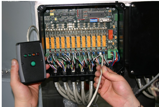
Figure 67 – Motor Control Handset plugged in the PDB
