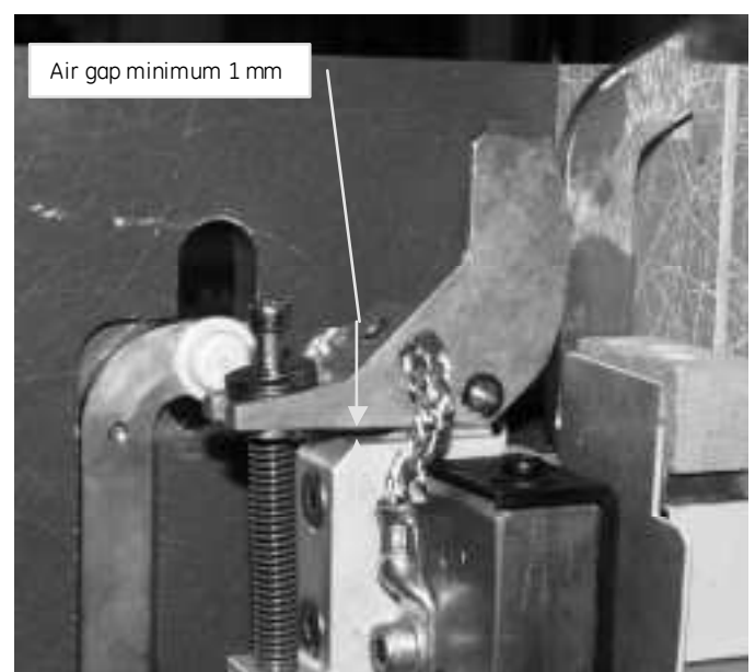
Fig. 47 Inspection of the arcing contact's air gap
