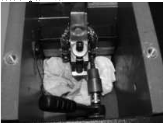
Fig. a Protecting of the arcing area against falling parts
