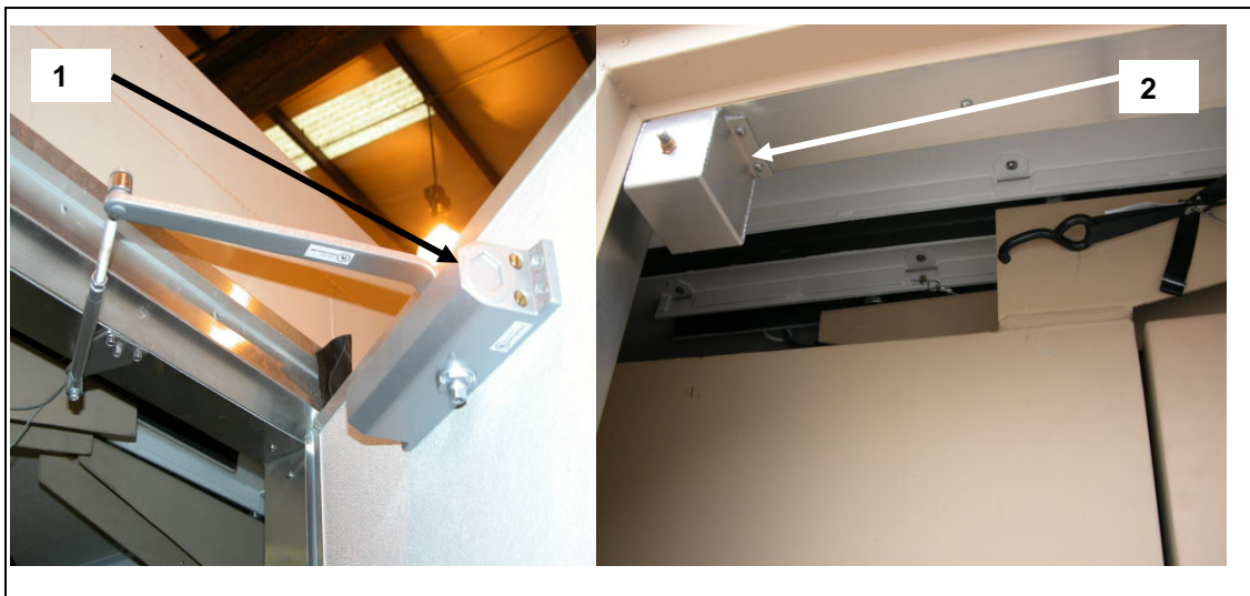
Figure 4.3-1 Door Damper and Door Light Switch
