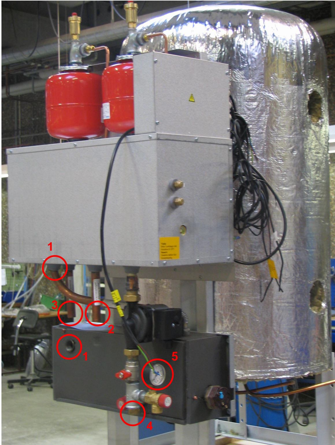
Figure 2: Ground source heat system without front panel.
