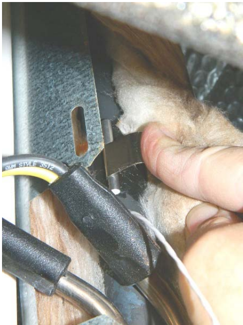
Fig. 4 Boiler Housing with Open Heater Access Door and RTD Clipped on
