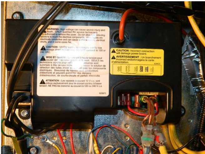
Fig. 12 Typical Norcold Power Terminals
