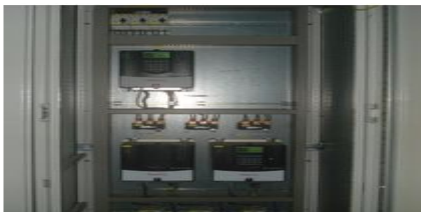
Fig. 5 Drive panel view for experimental set up
