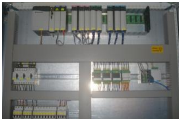
Fig. 6 PLC panel view for experimental set up
