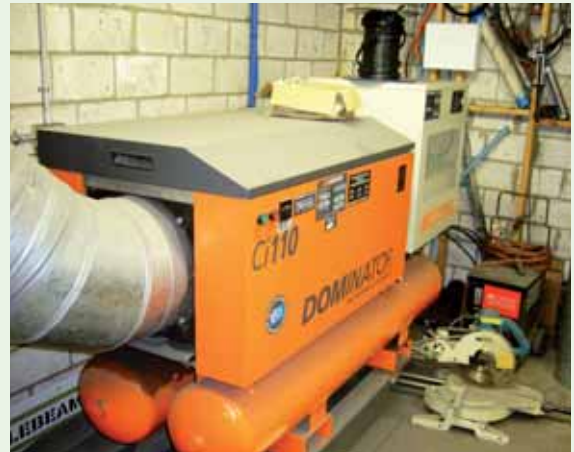
Well maintained air compressor
