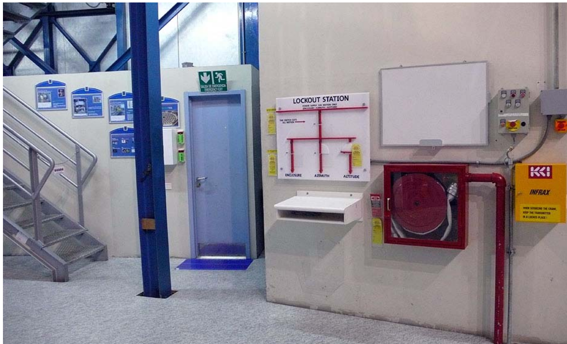
Figure 14 Lock-out station located on the azimuth area of each UT where a new lock-out switch will be installed to interlock the laser during work in the Nasmyth adaptor or in the Coude optical train
