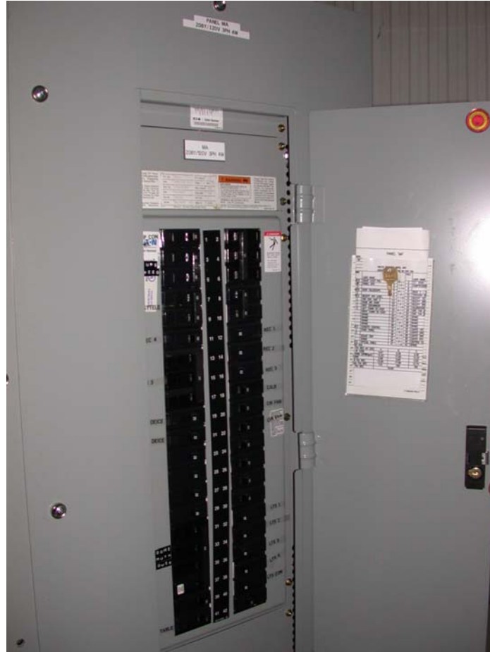
Power Distribution Cabinet
