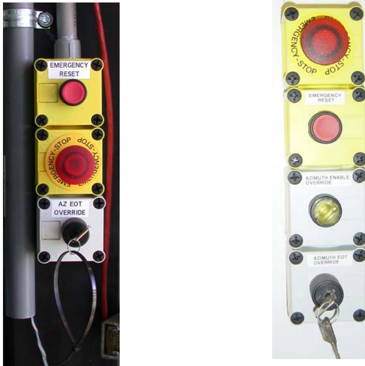
ESTOP and ERESET Buttons on Level 1: Typical Installations
