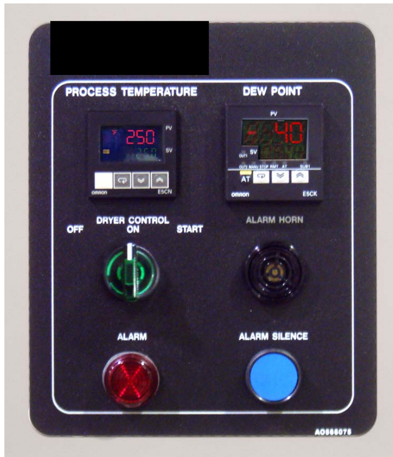
Figure 8: Typical Dryer Control Panel
