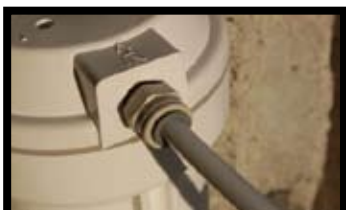
SIDE VIEW OF FILTER HOUSING
