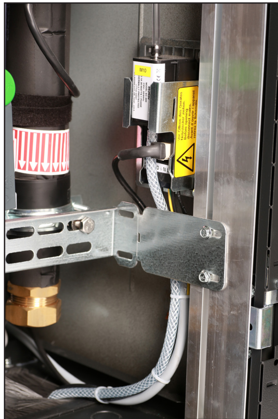
Condensate pump location
