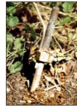
Grounding rod in the earth
