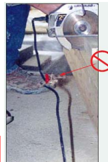
This cord has been spliced using a wire nut. Spliced cords are very dangerous!
