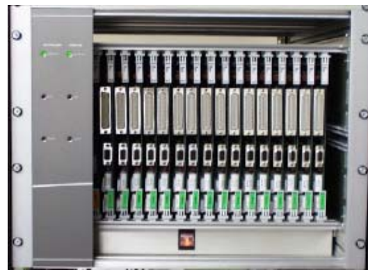
Fig. 3 Mainframe 6000 (door removed)
