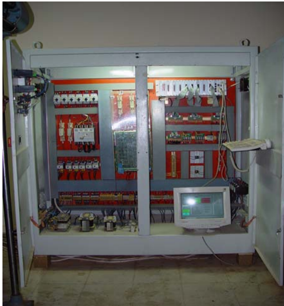
Figure 8: The new control cabinet
