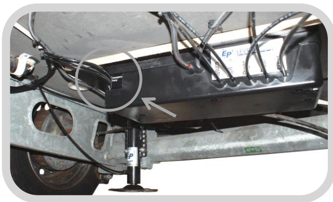
Protective pump housing with the connections to the emergency pump.
