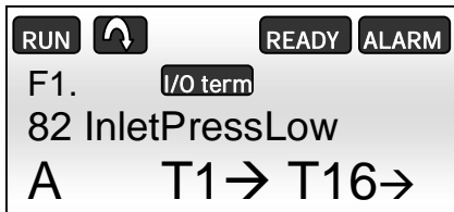
Figure 5.1-4, Low pressure alarm on the NXP panel
