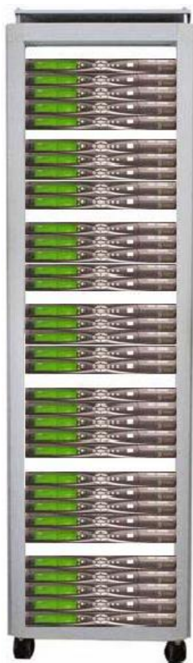
Figure 2-2: Encoders Mounted in a Single Rack
