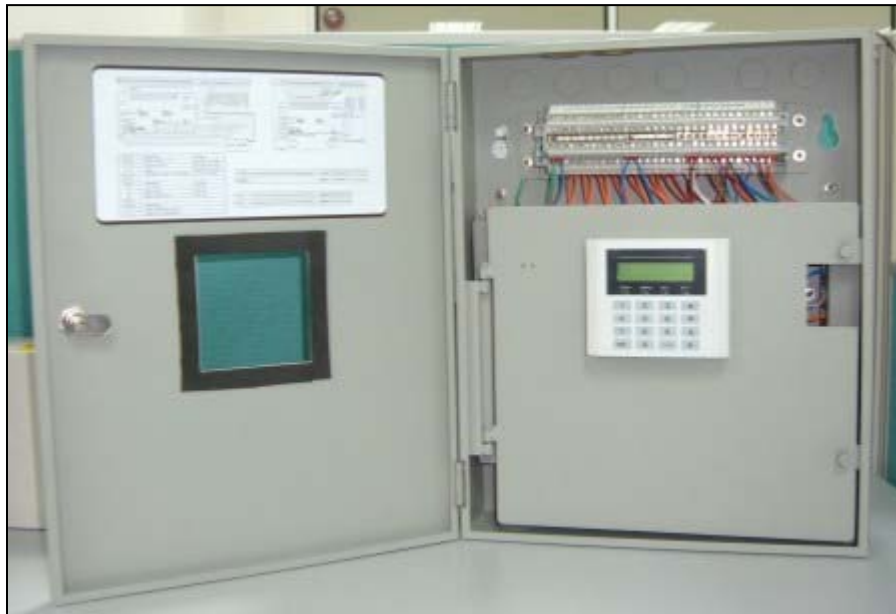
Figure 1: Loop Water Controller Internal View
