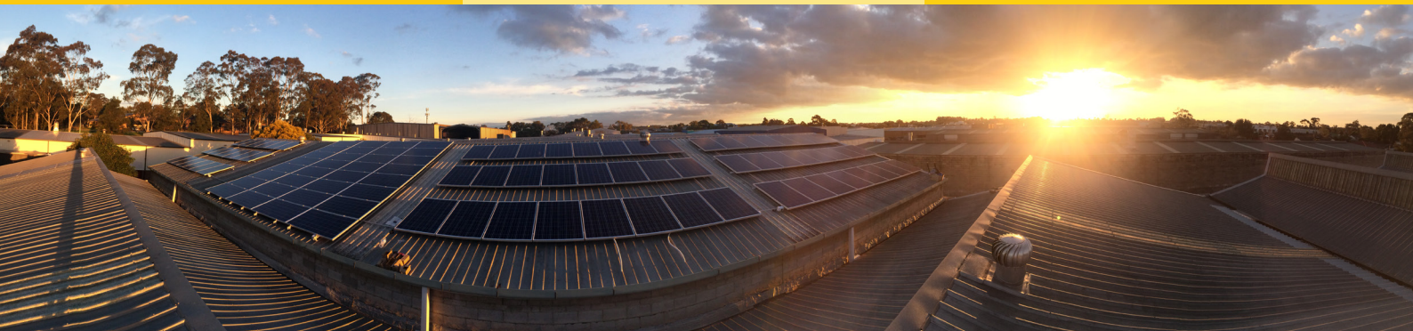
Girraween NSW 25 kW system June 2014
