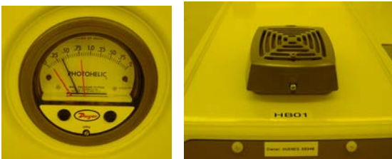
Figure 3. Photohelic Exhaust pressure gauge (left), and alarm horn (right)
