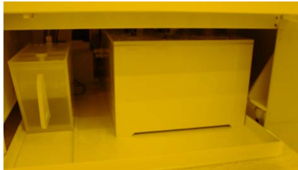
Figure 7. Catch tank (Right) and Caustic Reservoir (Left) under the hood.
