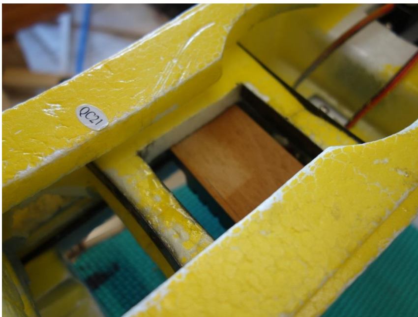
View from underside indicating openings introduced and the underside of the sound module support ply plate
