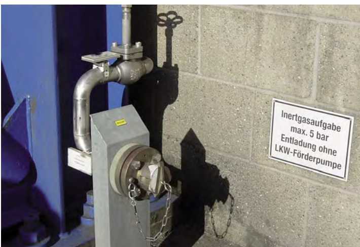
Picture 9: Inert gas connection to stationary evaporator
