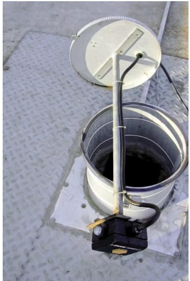
Picture 4: Smoke detector in a practical application
