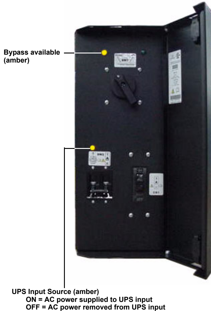
Figure 4 Maintenance Bypass Cabinet in Bypass Mode
