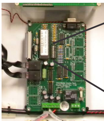
View of the master board showing location of the Dip Switch
