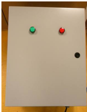
Control unit with door closed
