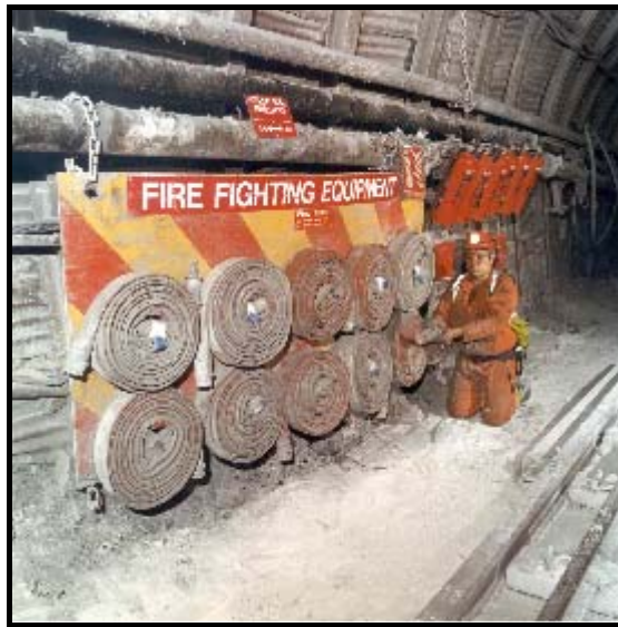
A well laid out and maintained fire point below ground in a coal mine
