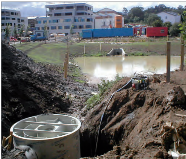
Installation of a Downstream Defender® to protect an attenuation pond from grits, silts and oils from the local road and domestic surface runoff. The discharge from the pond is controlled by a Hydro-Brake® Flow Control.
