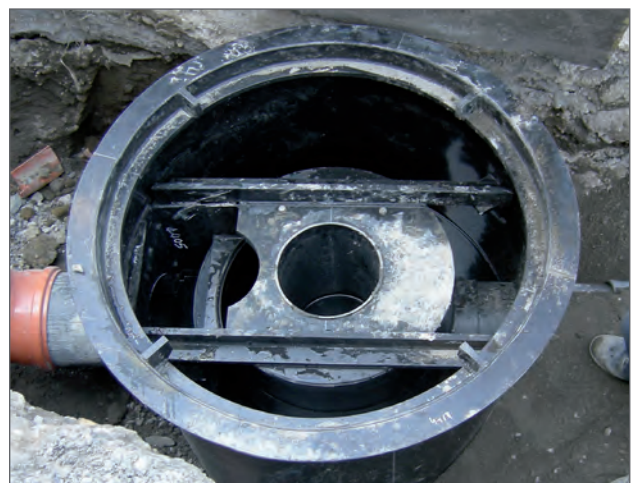
HDPE internals fitted to a reinforced HDPE chamber.
