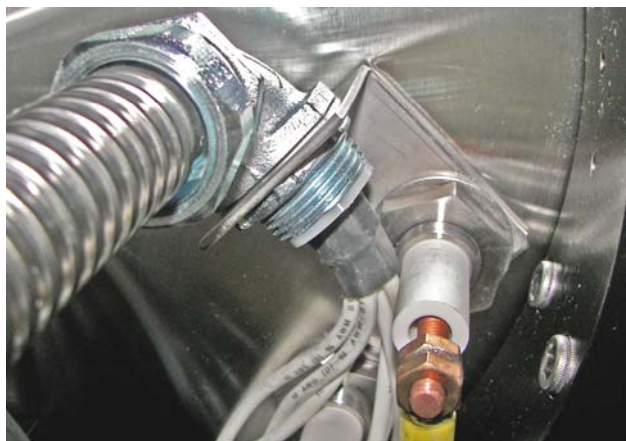
Figure 2-10 HV Conduit Bracket Properly Installed on HV Feedthrough
