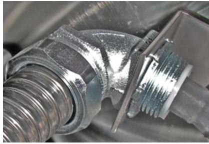
Figure 2-11 HV Conduit Properly Secured to Bracket
