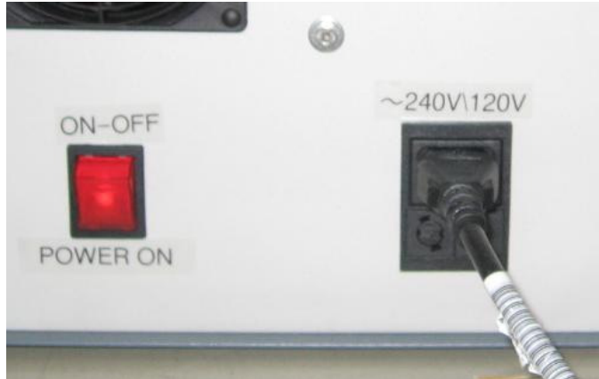
Figure 10: Main power line connection (supply unit back)
